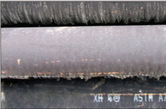
Tar coated cast iron pipe
